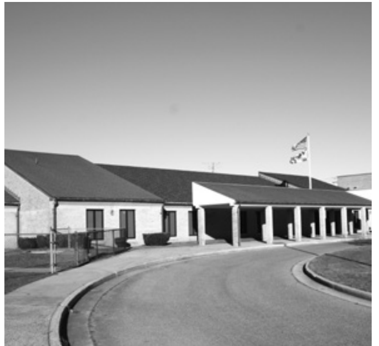
Improvements needed by the Emmitsburg Elementary School include replacing the existing heating, ventilation & air conditioning systems, and replacing the roof and flooring.
