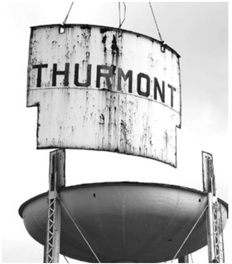
The old Thurmont water tower was built in 1939, but has been out of service for the past 10 years.
