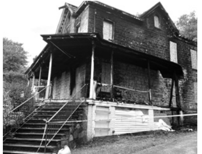
In spite of Herculean efforts on the part of multiple fire companies, the 100+ year old rectory was completely destroyed.
